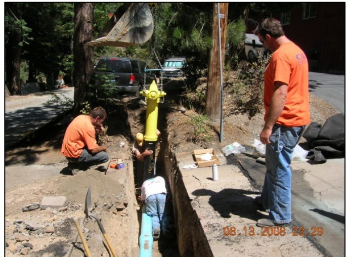
Installation of New Waterline in the Street (Photo courtesy of North Tahoe PUD)
